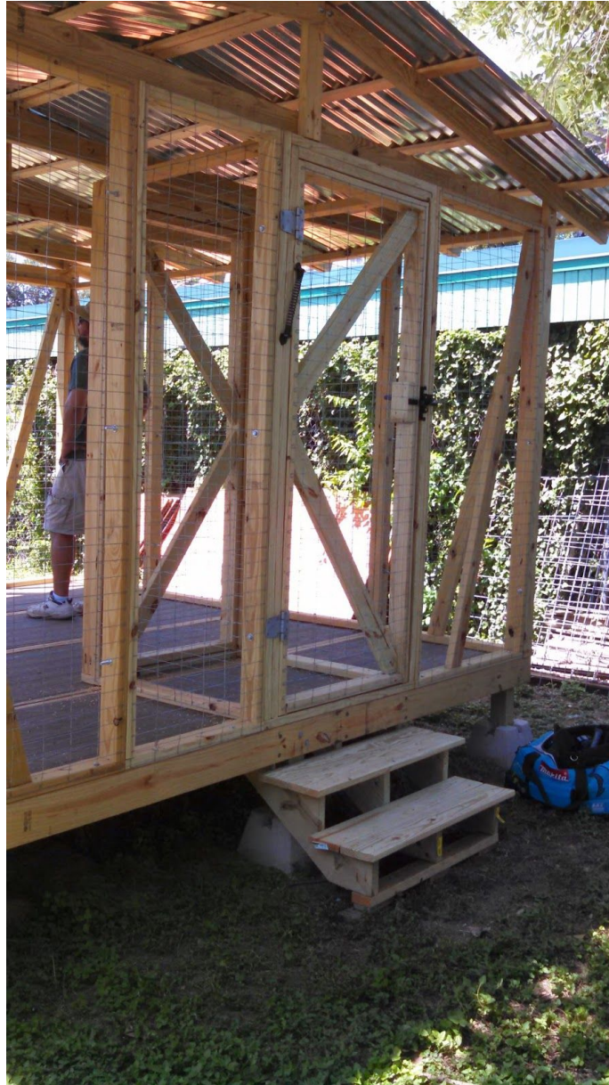
Photo showing modular sections, airlock and stairs.. Photo was taken before second layer of wire screening was added.
