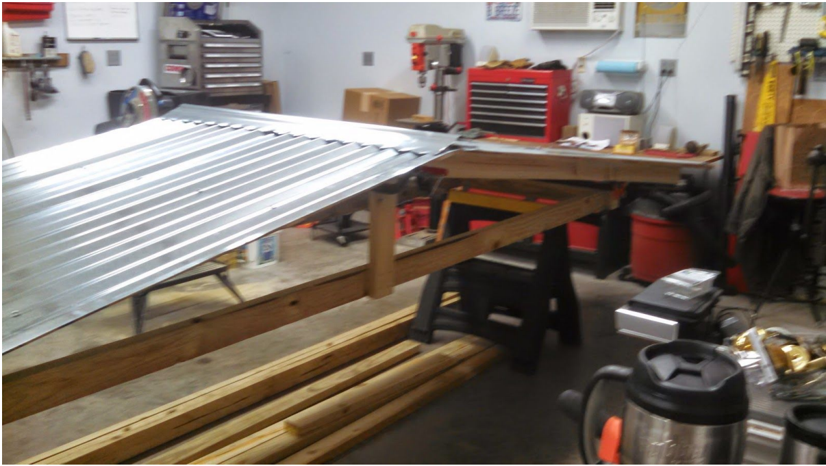
Photo showing an end pair of roof panels under construction. Note king post and truss bottom component.
