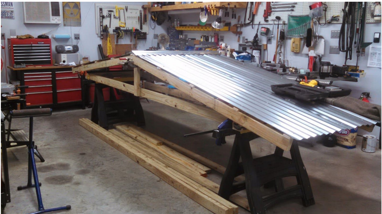
Photo showing back side of roof module pair (interior side) plus king post and truss bottom.
