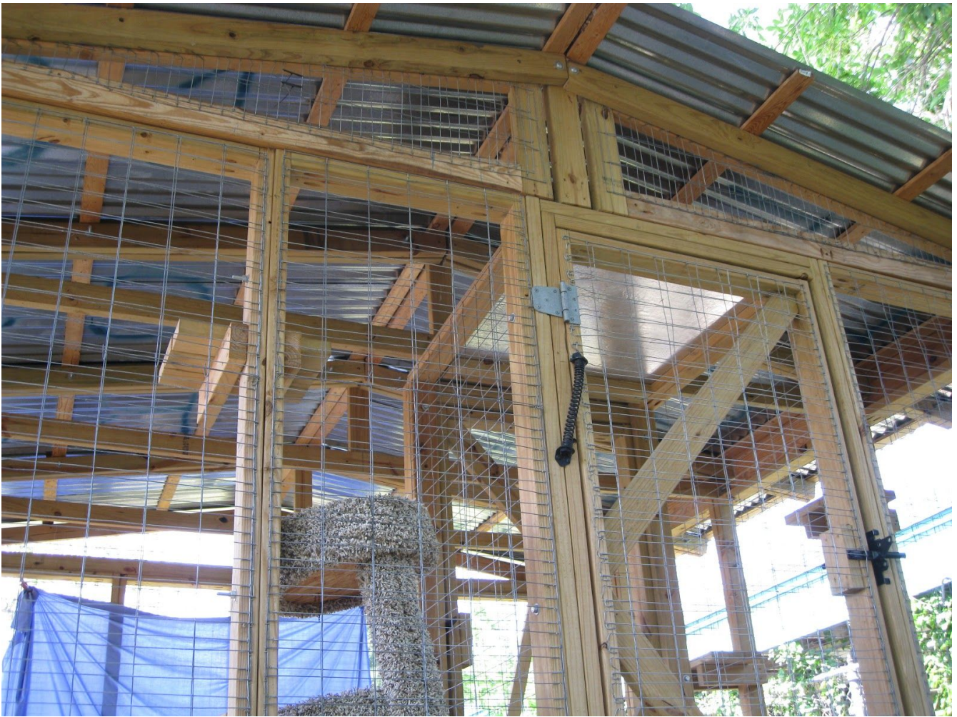
Photo showing door, rafter and top screen details. Note that smaller module is to the left of the door module.
