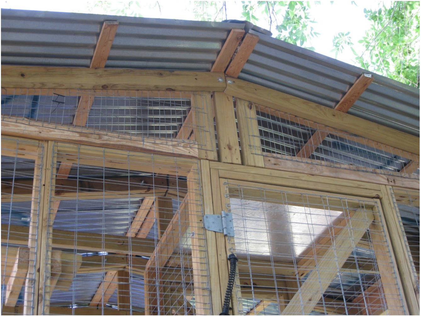
Photo showing roof modules, top screens and door module. Note plywood attached to top of airlock.
